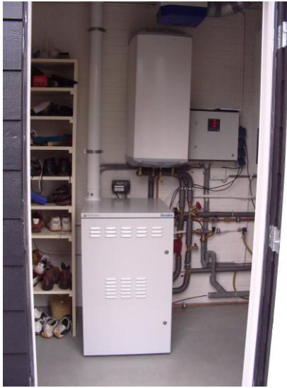
Figure 4-3: The CFCL BlueGen installed in an installation room. De CFCL BlueGen stands on the floor and there is a 100 liter warm water storage on the wall.
