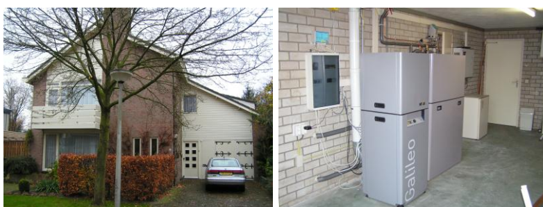
Figure 4-1: Field test location and installation room Hexis Galileo 1000N
